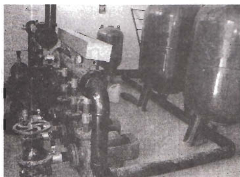
i. Booster pumps and Pressure Tanks
